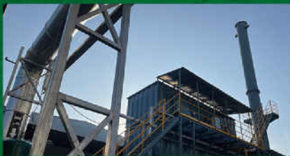
RTO-Waste Gas Treatment System
