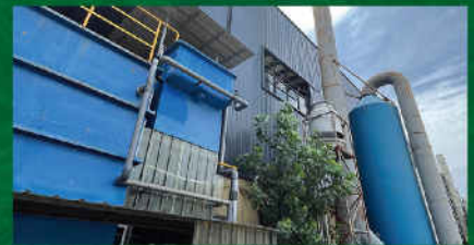
Waste Water Treatment Station
